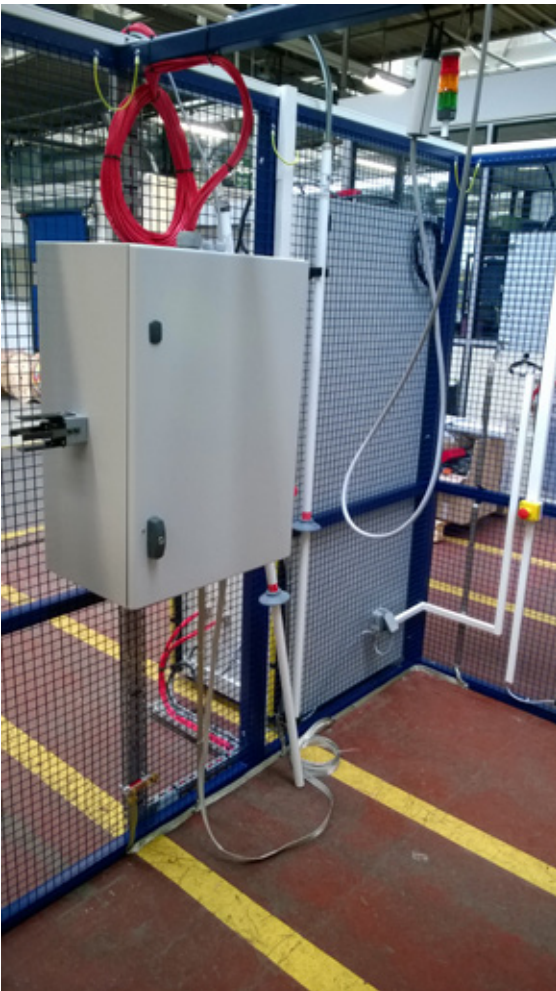
Connection interface and safety grounding stick
