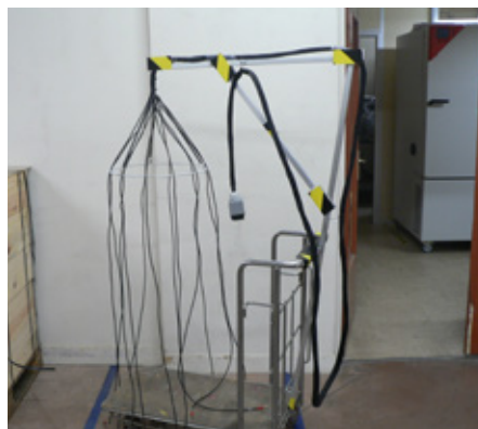
Connection harness installed on a bracket
